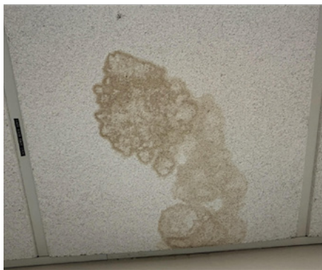
Ceiling in need of improvements and asbestos abatement.
