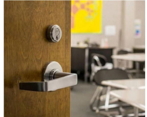
Door hardware needs replacement.
