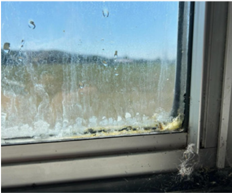
Windows need replacing for efficiency and safety.
