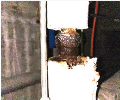
Plumbing infrastructure is aging and deteriorating.
