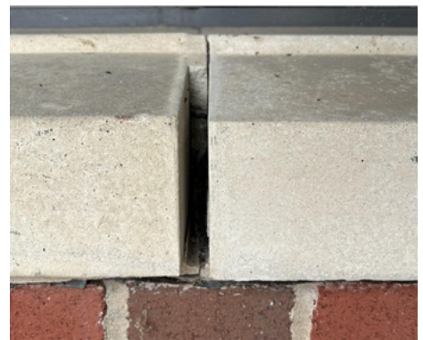
Masonry in need of restoration and repointing.
