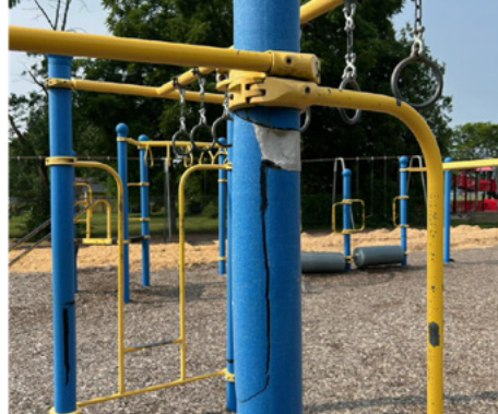
Playground equipment is deteriorating.
