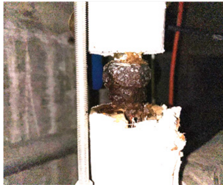
Plumbing infrastructure is aging and deteriorating.
