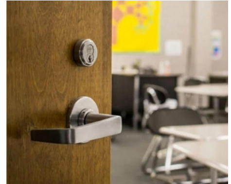
Door hardware needs replacement.
