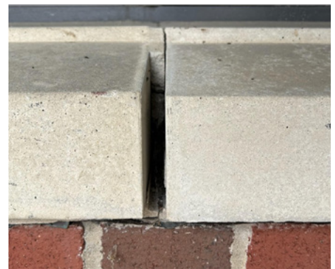
Masonry in need of restoration and repointing.
