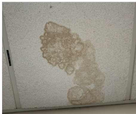
Ceiling in need of improvements and asbestos abatement.
